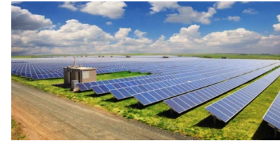
NorthStar Clean Energy – MISEC Choice Solar Farm
